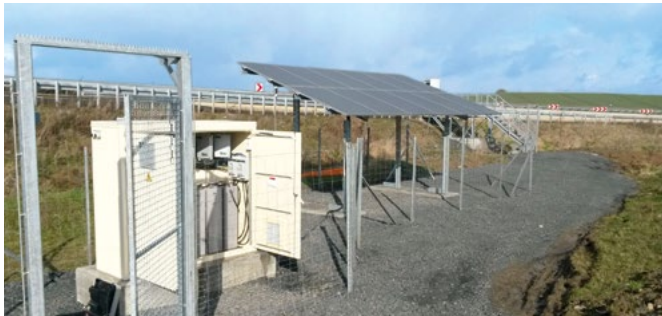
Power supply of a measuring station for speed control
