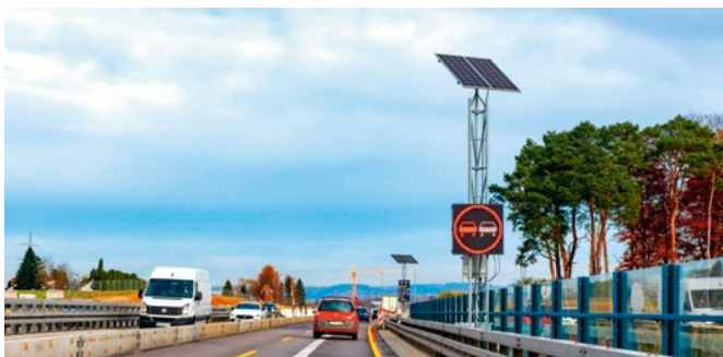
LED road sign
