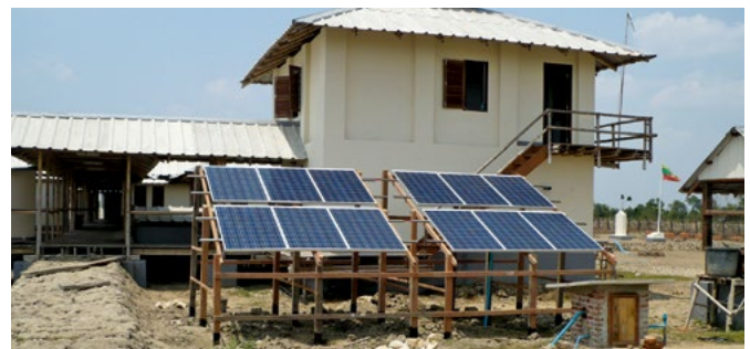
Power supply to a hospital
